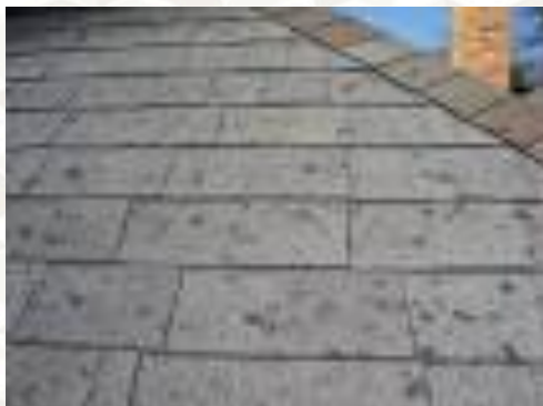
Damage to Asphalt Shingles
