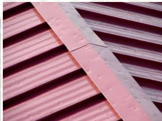
Damage to Metal Roof
